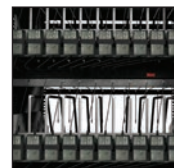
POWER BRICK LACING
